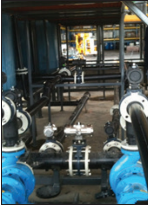
HYDROFRACTURING CHEMICAL BLEND PLANT
